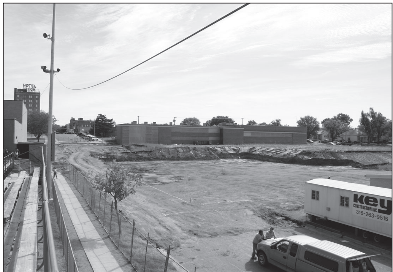
The building site for the new high school begins to show signs of progress. Pratt High's new building is due to be completed in 2007. Photo by: Neil Goss
